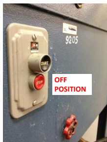
Figure 2. Main power in OFF position. Red STOP button compressed.
